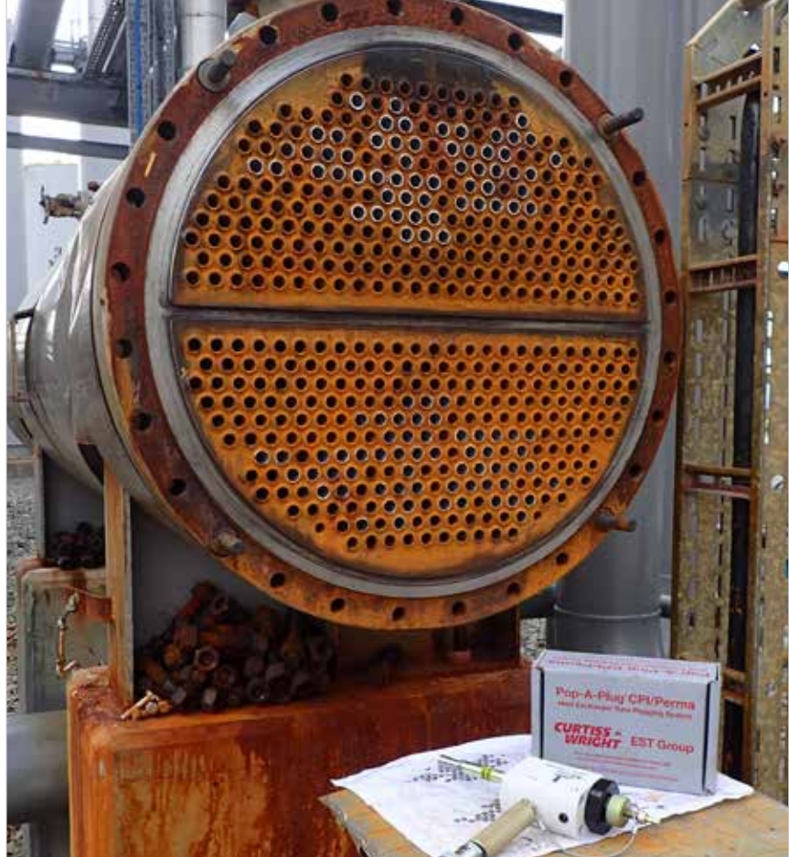
Pop-A-Plug Tube Plugs saved approximately 75 hours of maintenance work
